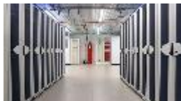
MODULAR DATA CENTER ENGINEERING
