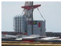
GENERATOR & ELECTRICAL BUILDINGS
