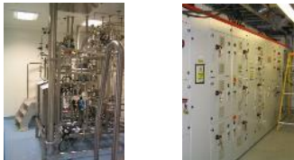
PURPOSE BUILT SOLUTIONS
