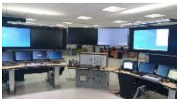
ONSHORE CONTROL ROOMS
